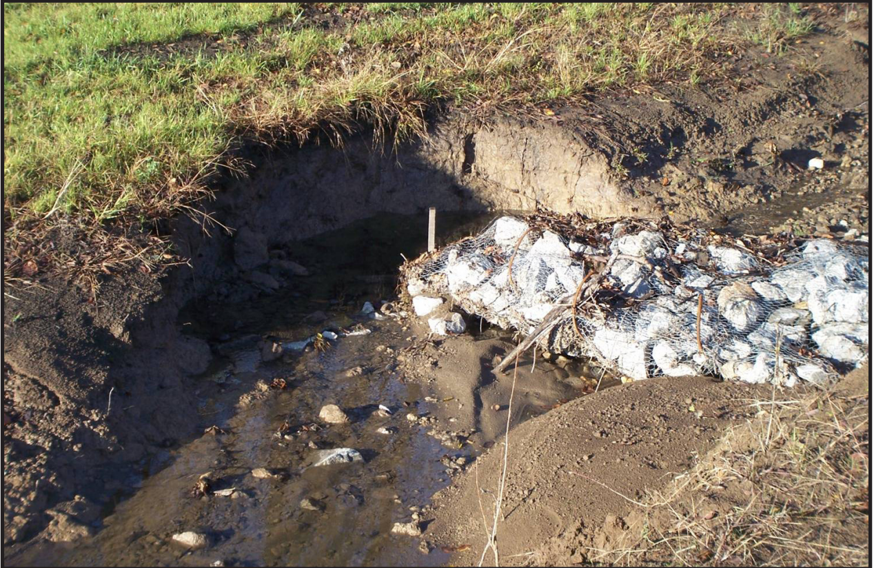
Figure 2.3 The improperly installed check dam created significant bank erosion. Source: ABC's of BMP's LLC
